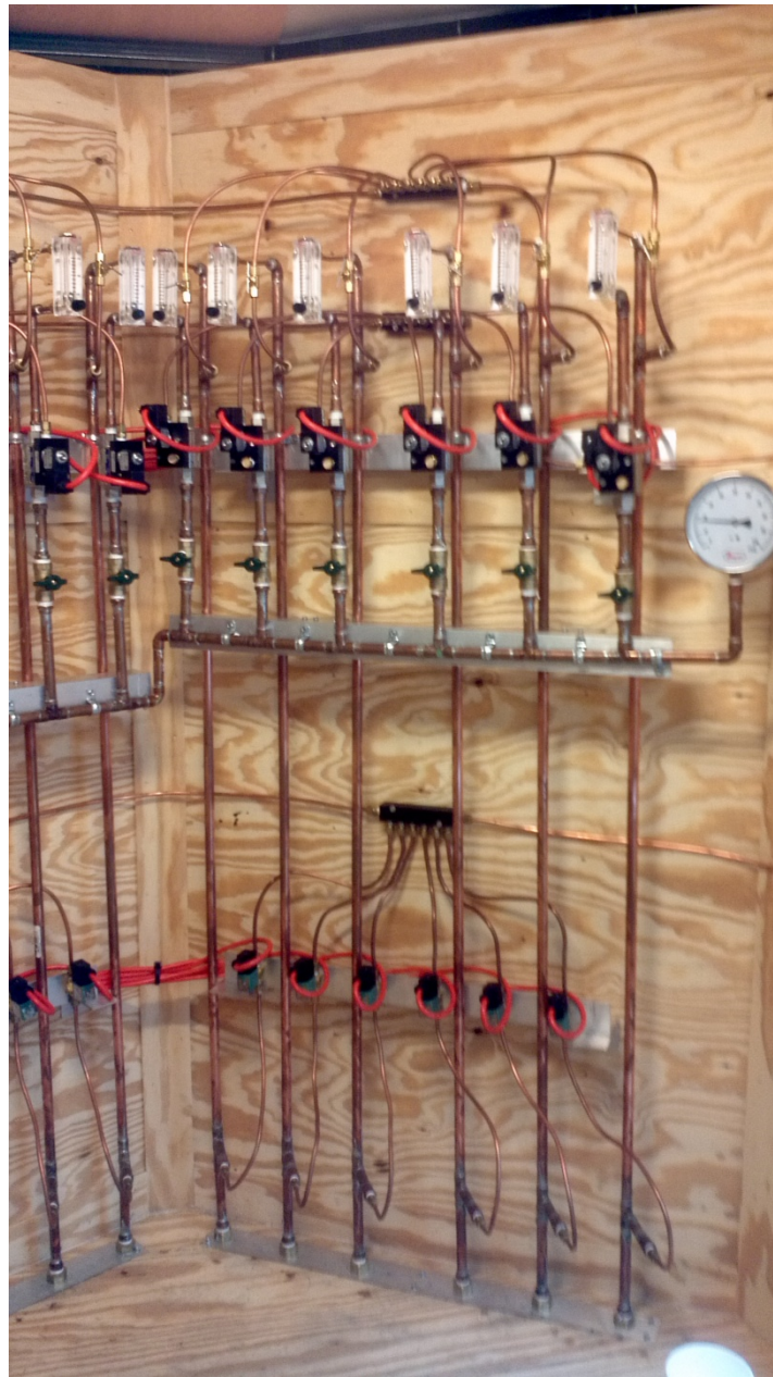
Six of the twelve injectors showing independent air flow control, nitrous oxide dosage on top and TEP dosage below.
